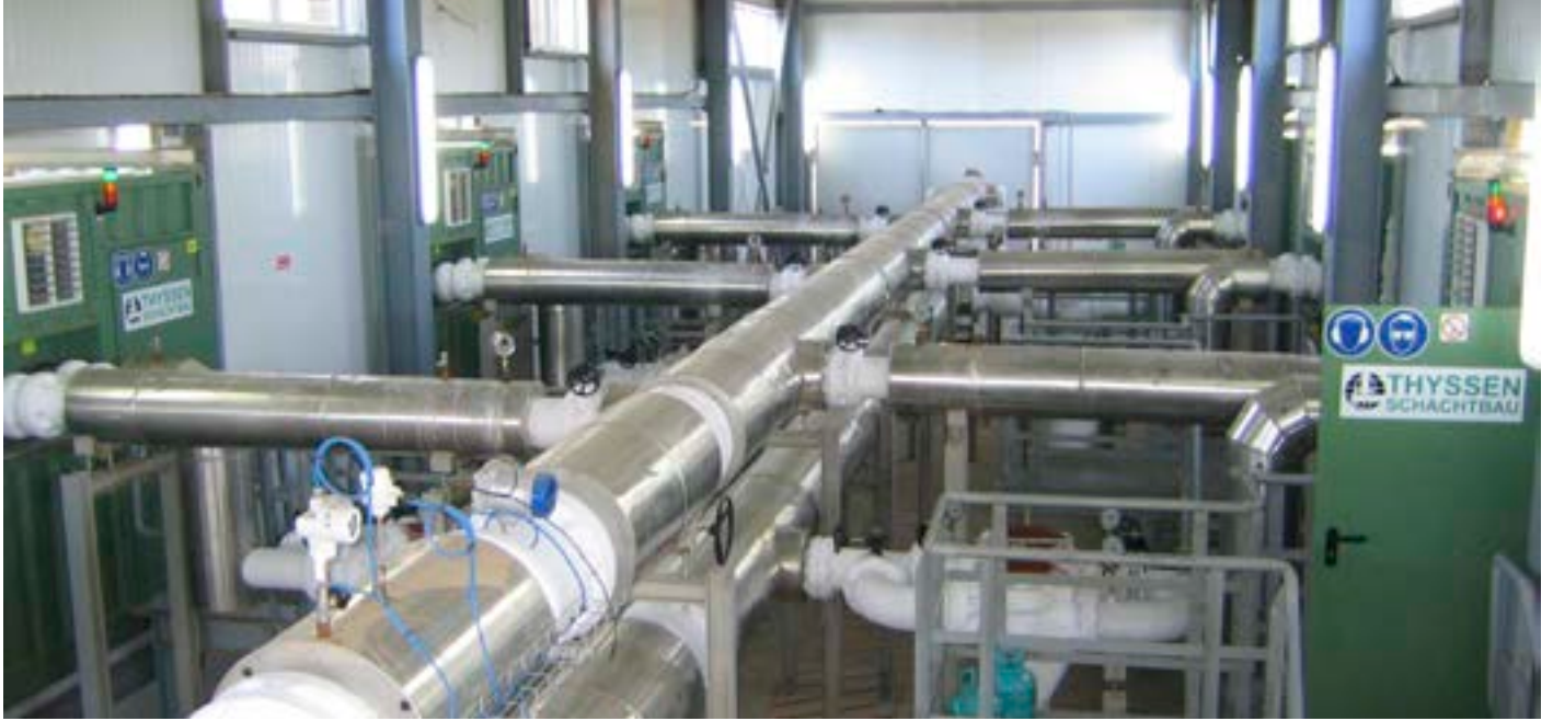
Massive pipelines branch off from the pump house to the individual containers where the freezing systems are located.
